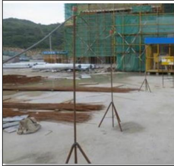
Lighting fixtures at night
