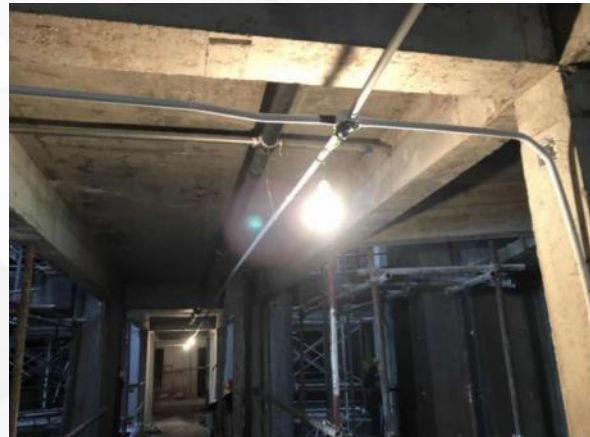
Temporary wiring at site
