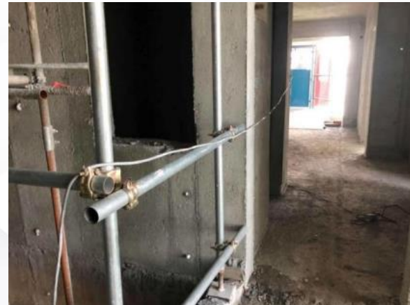
Electrical cable hanging to avoid soaking in the water and tripping hazard
